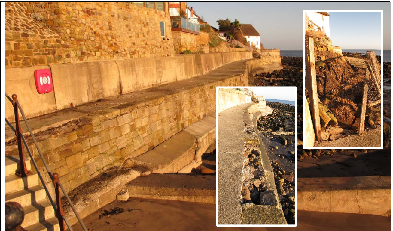
Runswick Bay Village seawall on 17 th December 2013 showing damage to blockwork following the storm surge incident of 5 th December 2013
